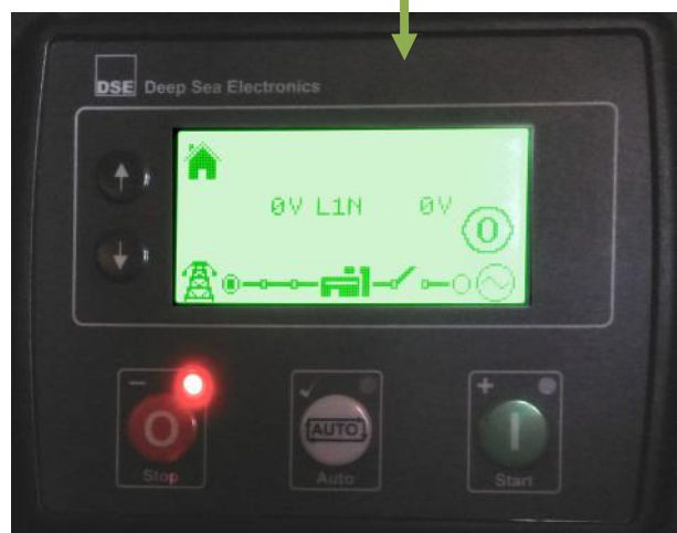
Control Panel powered ON
